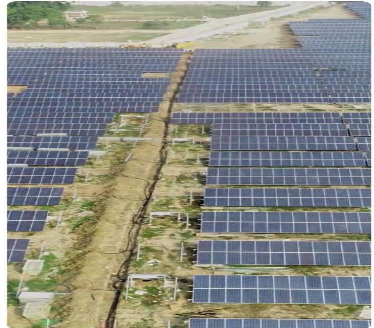
Solar Power Plant at Manuguru (30 MW)
