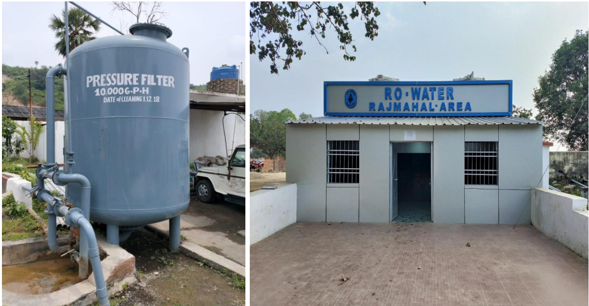
Figure 7.3: Pressure Filter and RO Water Facility at Rajmahal Area, ECL
