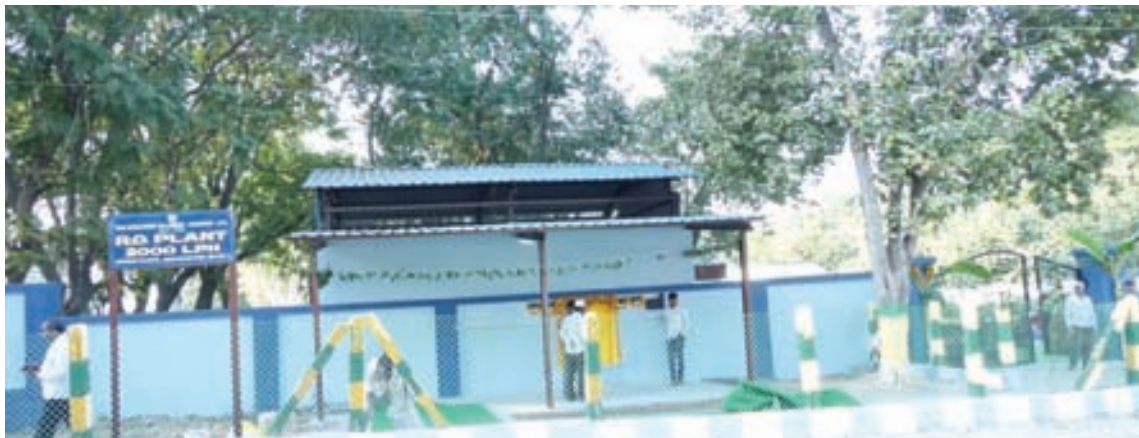
RO Plant - 2000 LPH at RG-1 Area
