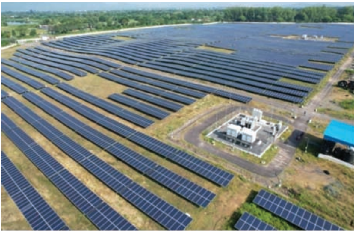
Solar Power Plant at Mandamarri
